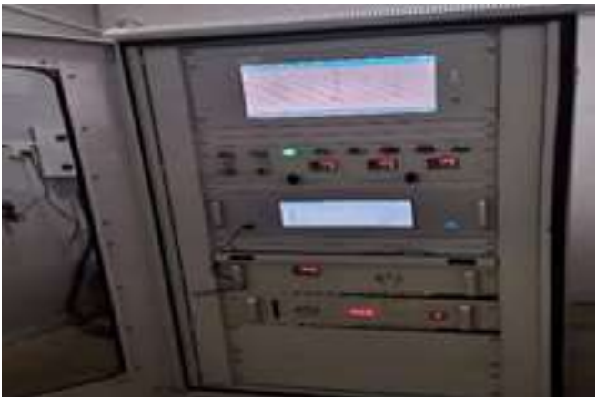
Online monitoring equipment
